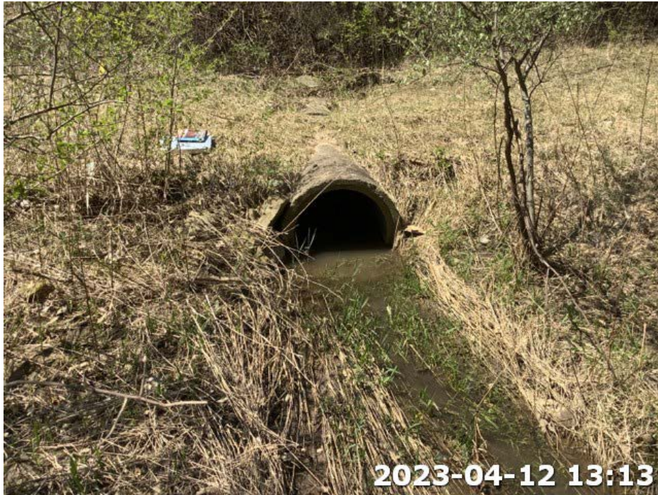
Photograph Location 14. View of existing culvert and downstream portion of Stream 1. Photograph taken facing upstream/west.
